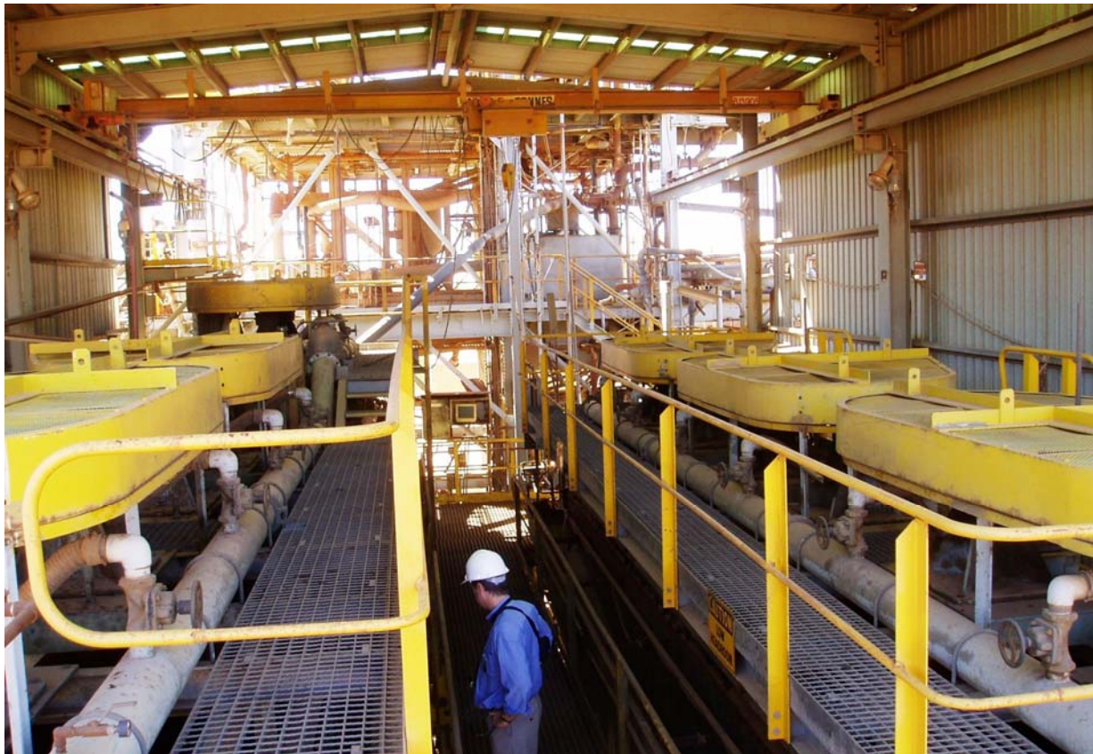
The flotation circuit acquired as part of the Telfer sulphide plant
