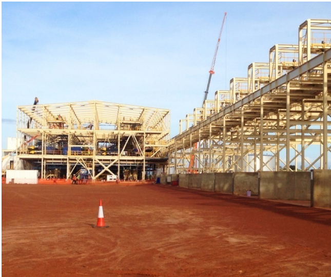
Wet Mill at MSP
