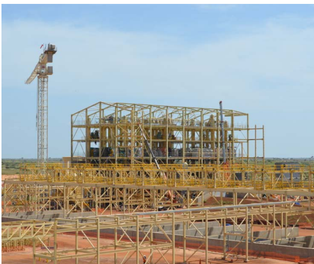
Intermediate non-mag concentrate storage & Dry Mill
