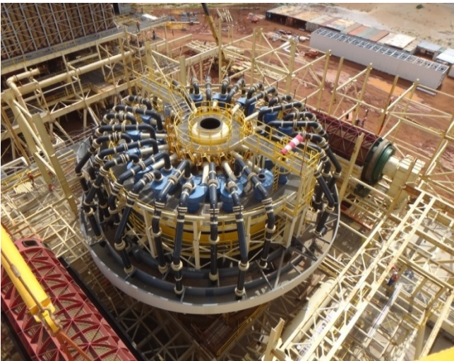
Surge bin cyclone cluster on WCP
