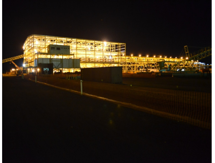
Night shift in action at Wet Mill
