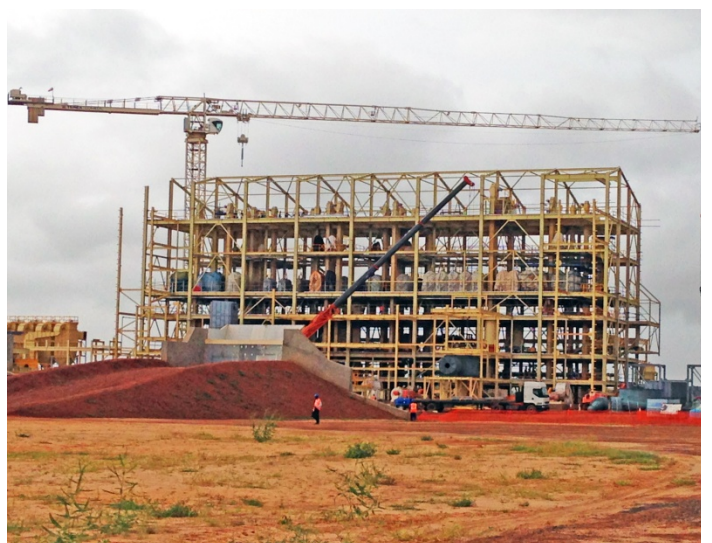
Dry Mill at MSP
