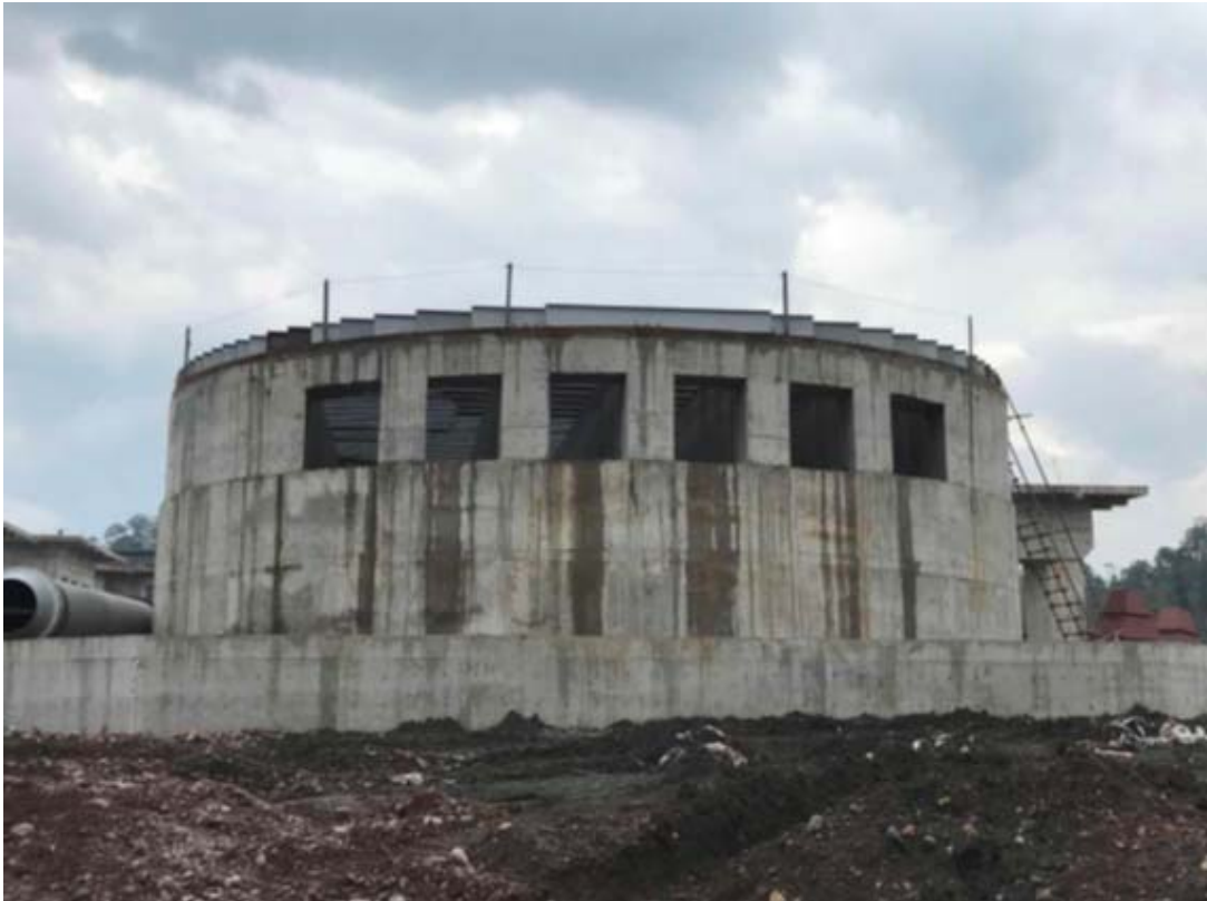
Base for Ranger Nickel electric furnace
