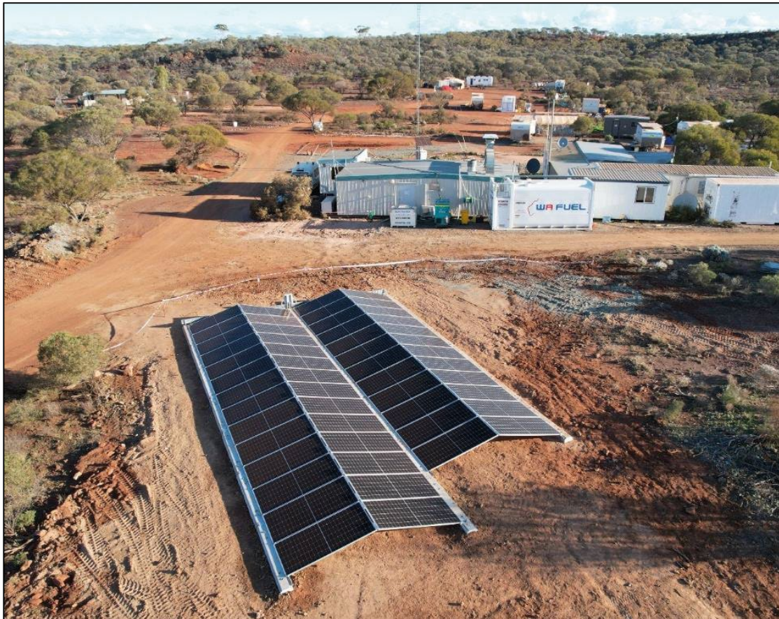
FIGURE 9; 20kW SOLAR FARM AND 98kWh BATTERY INSTALLATION TO PROVIDE ENERGY FOR THE MT IDA CAMP
