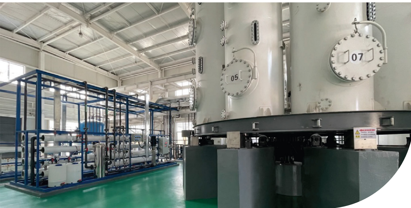
Figure 3: Lanshen DLE test facility in Xian, China
