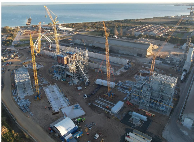
Current Progress photo of Kwinana Cockburn Cement upgrade – performed by SIMPEC under a LNTF
