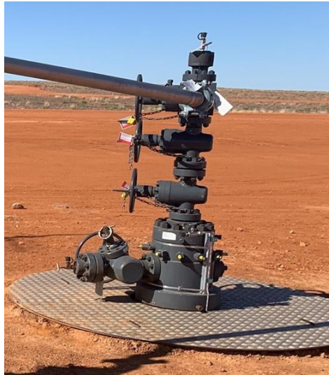
Figure 5: Wellhead at Yarrow 3 (Courtesy of Santos)
