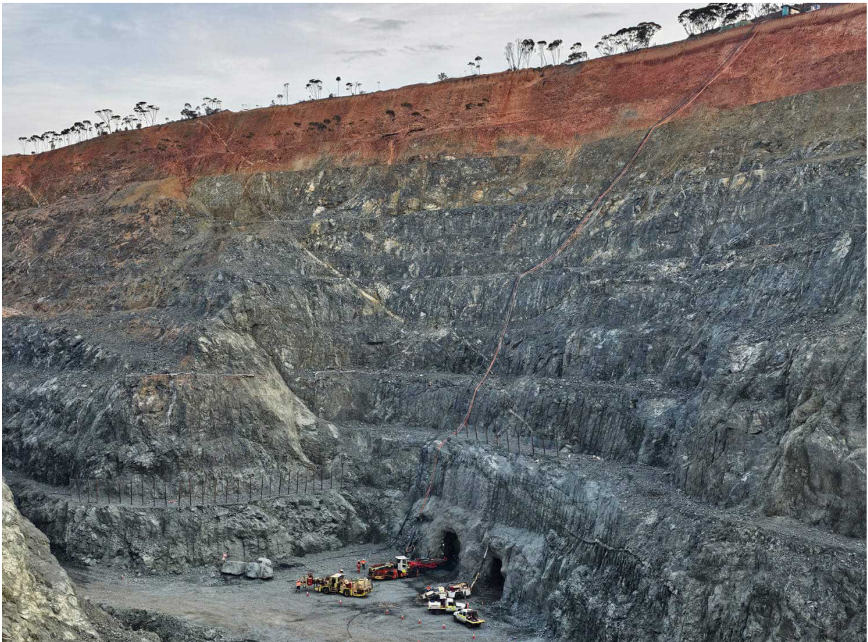
Picture: Scotia Underground Access and Fresh Air Portals
